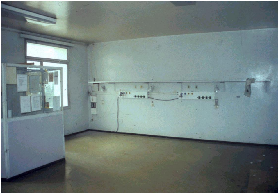
Picture 4. Wall-mounted distribution manifolds for oxygen, compressed air and electricity (1997).
