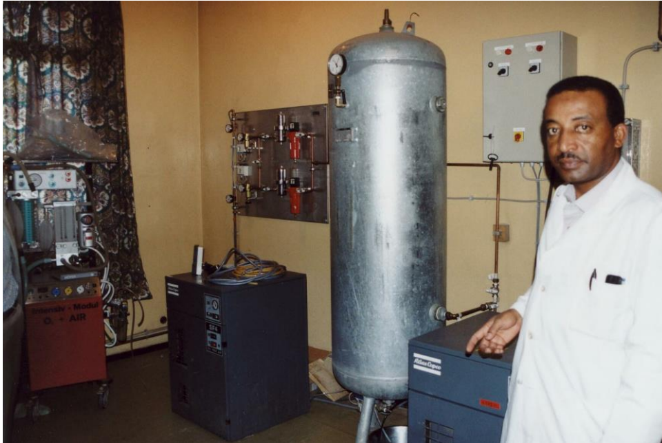
Picture 6. Duplex compressor system, compressed air buffer tank, filter assembly and switching unit together with Dr. Kinfu of the Black Lion Hospital.
