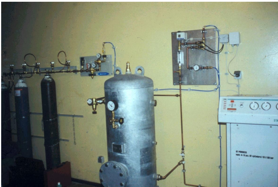
Picture 5. Oxygen concentrator, buffer tank and reserve cylinders (1999).
